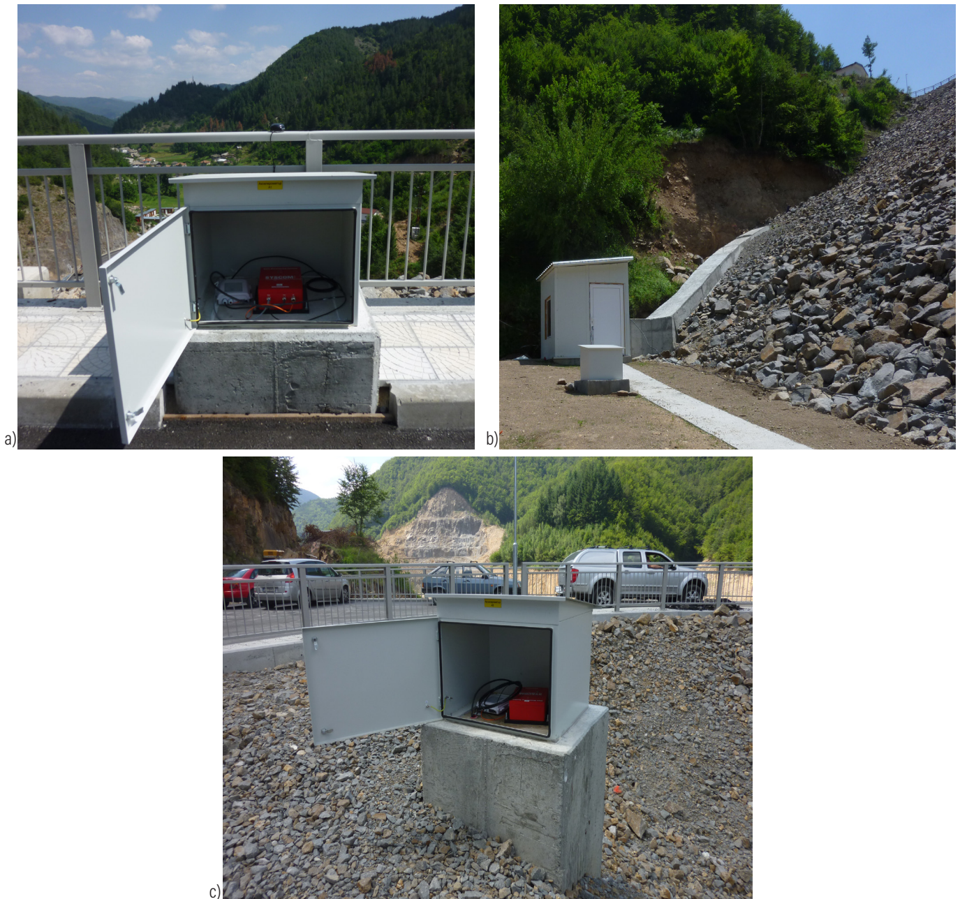
Figure 3. MR3000DMS instruments installed on the Plovdivtzi Dam: A1 (a); A2 (b) and A3 (c).
