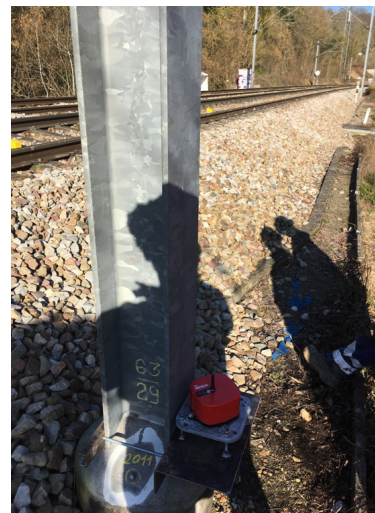
Figure 2. ROCK installed on a catenary pole
