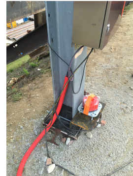
Figure 5. ROCK beacon close to the electrical box
