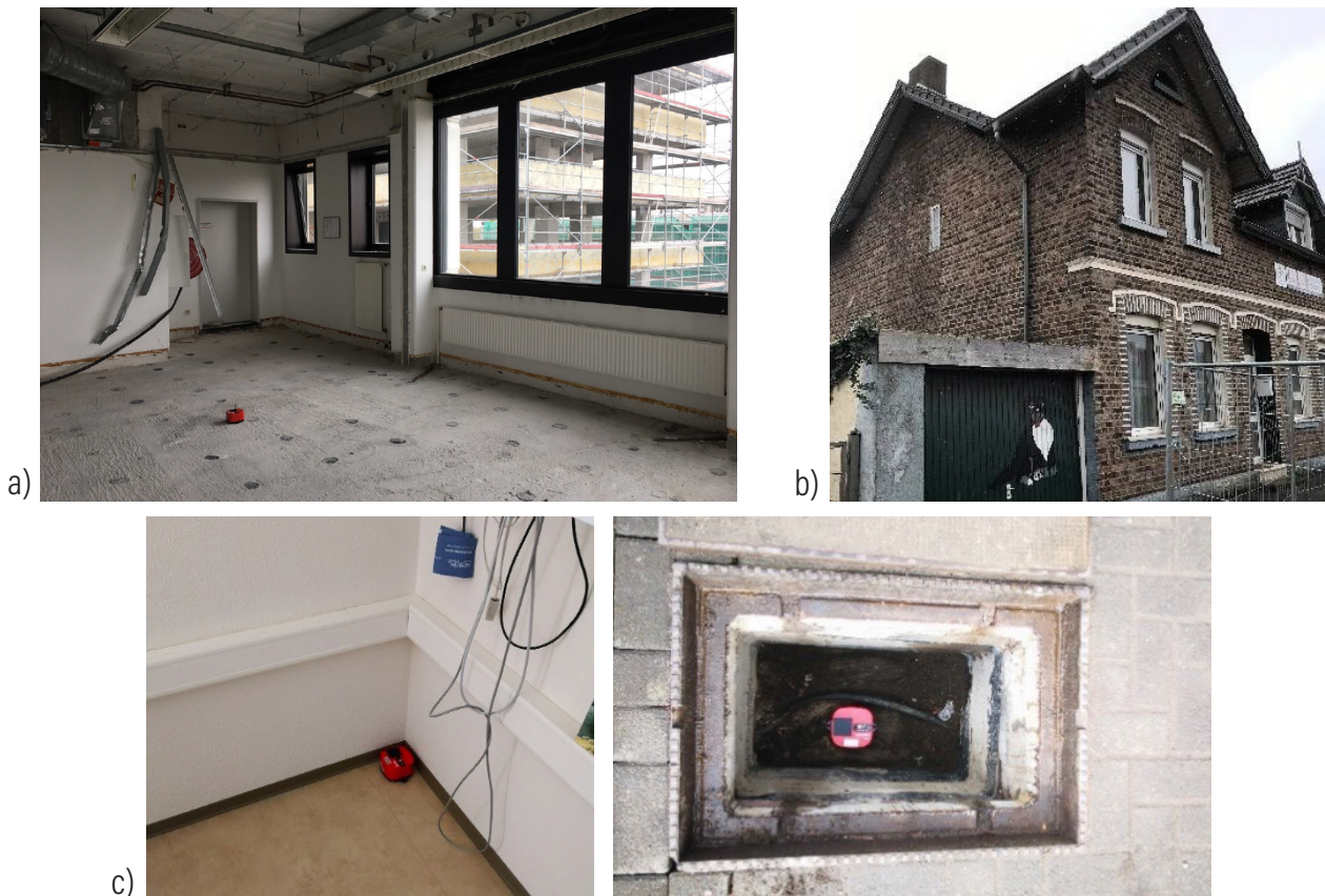
Figure 2. Real installations of the ROCK: a) in the vacant building close to the demolition monitoring; b) at the top of a house close to piling works; c) in the sleep clinic and inside the cable pit, for the monitoring of the construction site.
