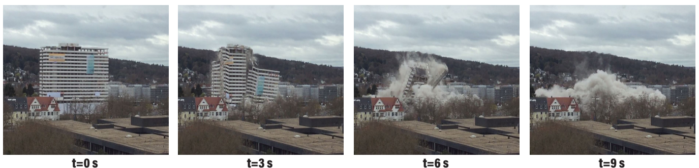
Figure 4. Successive instants of the Bonn Center demolition, seen from the Bonn Marriott Conference Hotel.
