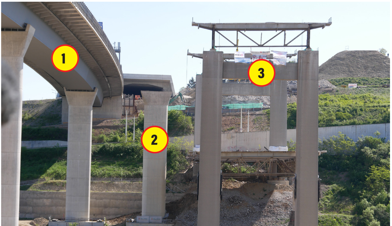
Figure 2. The northern carriageway of new bidge (1), the pier "70-Süd" (2) and the old bride (3) on the highway BAB A3 in Heidingsfeld, Germany.
