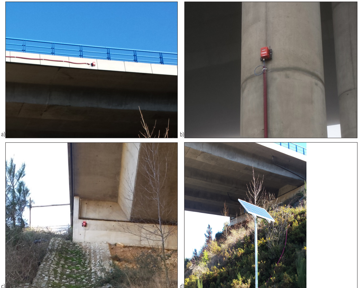
Figure 3. Instruments installed for the vibration monitoring of the A7 viaduct: a) MR1 on the external side of the bridge deck; b) MR2 on a pillar; c) MR3 on the bridge abutment; d) solar panel and battery for the power supply of the MR3000C devices.
