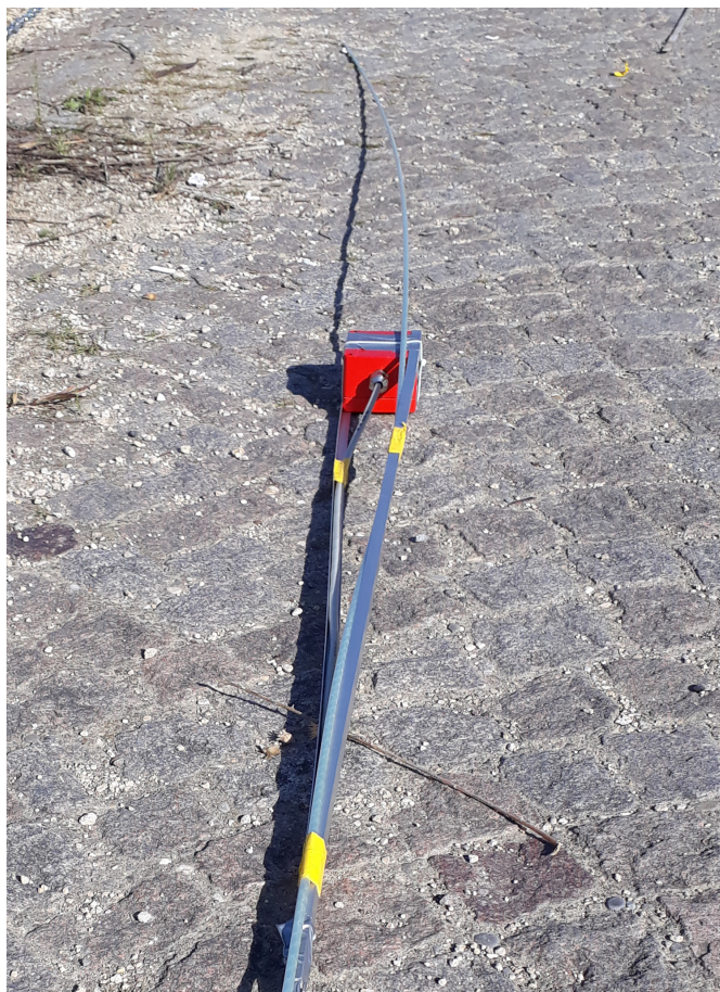
Figure 3. Borehole sensor ready to be inserted in the ground.
