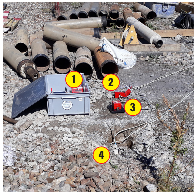
Figure 4. Measurement point MP1. 1) The recorder MR3000TR. 2) A junction box for the connection to the three external sensors. 3) The sensor at the surface. 4) The underground sensors.
